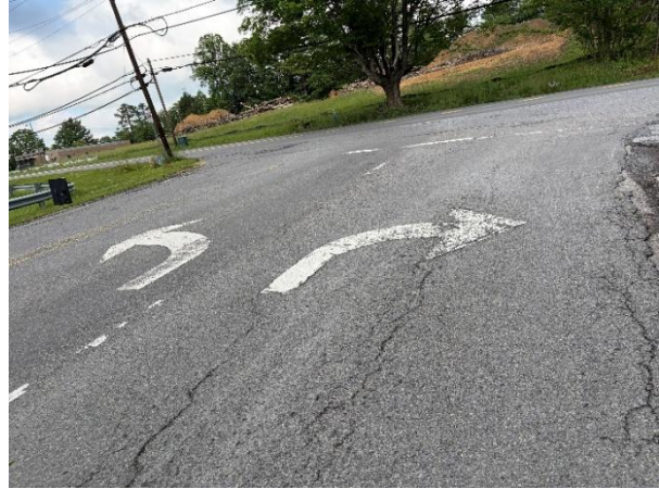
Photo 3: Faded Pavement Markings on Woodcrest Drive
