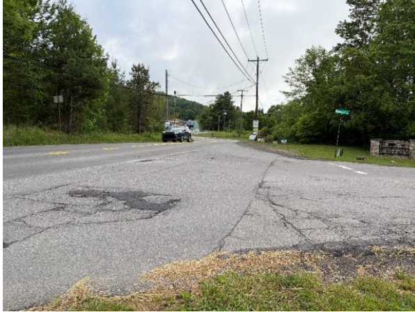
Photo 2: Deteriorated Pavement on Woodcrest Drive
