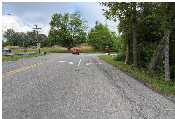
Photo 5: Deteriorated Pavement and Faded Pavement Markings on Woodcrest Drive
