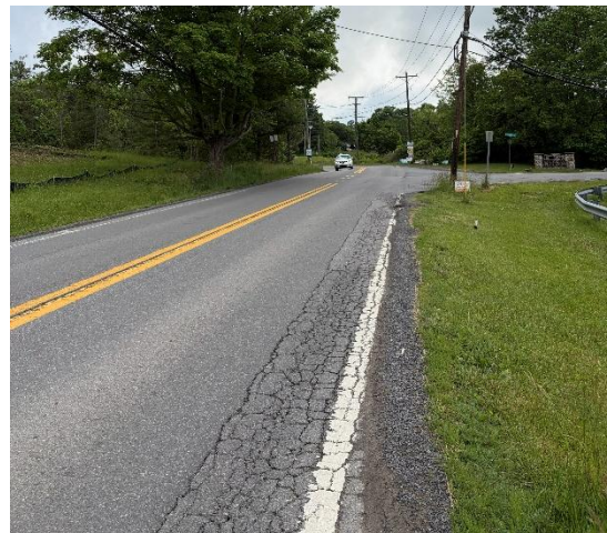
Photo 1: Deteriorated Pavement on Stanaford Road
